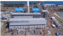
GLP Main plant
